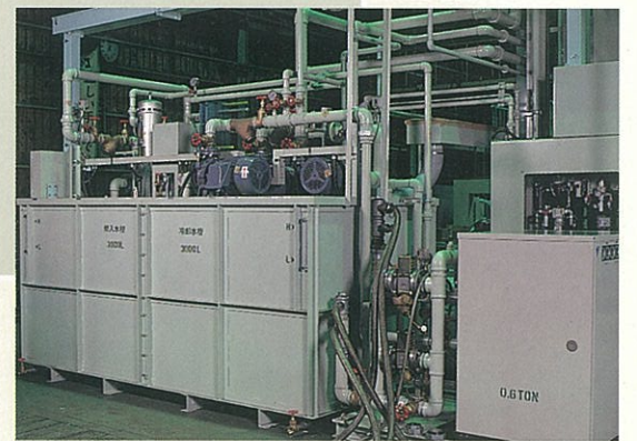
6 冷却水循環装置 Cooling and quenching water recirculation system
