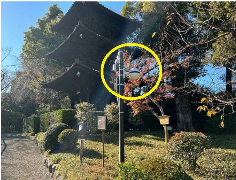
A Wi-Fi access point set up in Hotel Chinzanso Tokyo's garden (a spherical type that does not interfere with the landscape)
